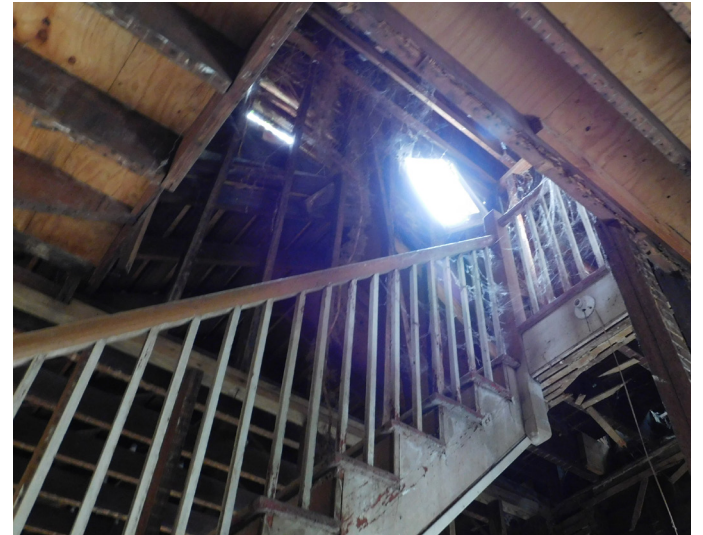
EXISTING NON-COMPLIANT STAIR
